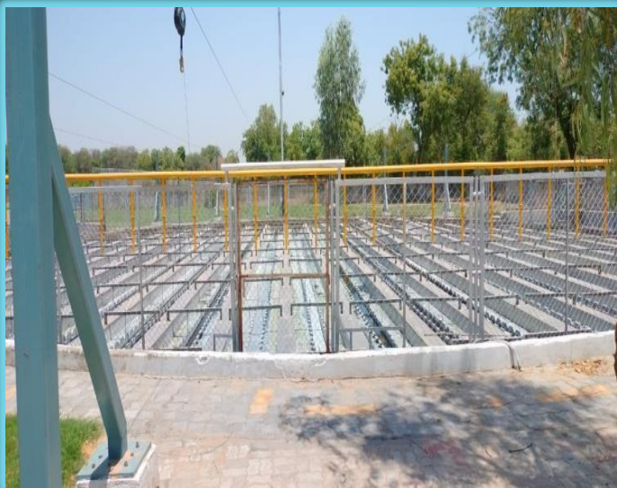
Biogas Generation in ETP
