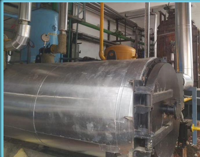
Hot Water Generator
